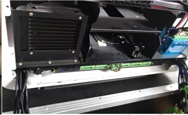
Green cables sorted out on two sides
